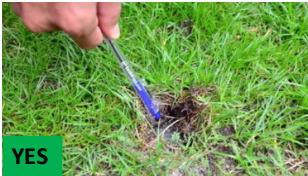
Concealed sprinkler head
